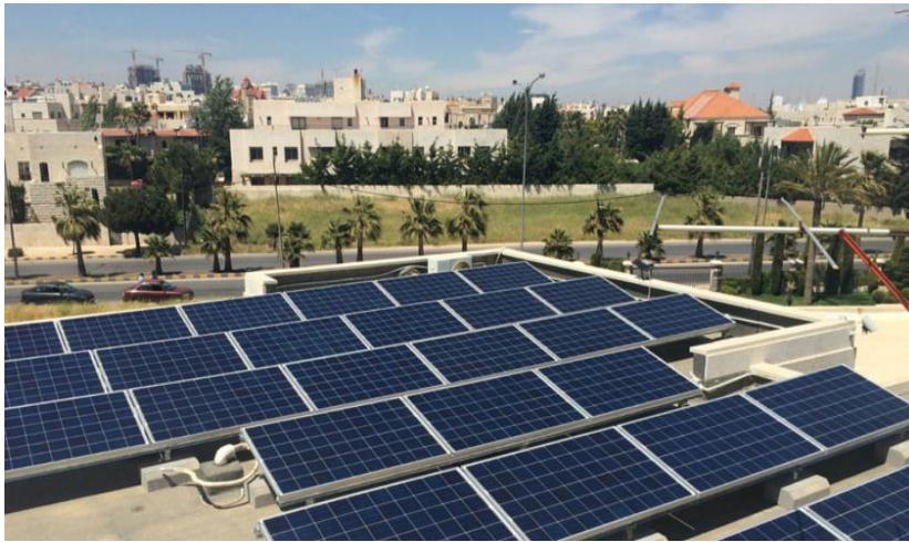
Residential Rooftop 10 kW – Amman, Jordan
